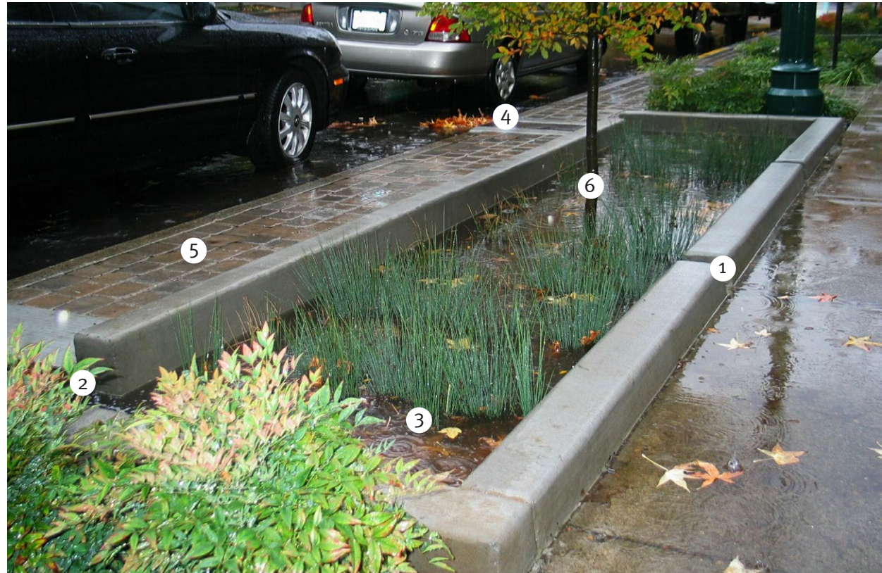
Bioretention planter in Portland
